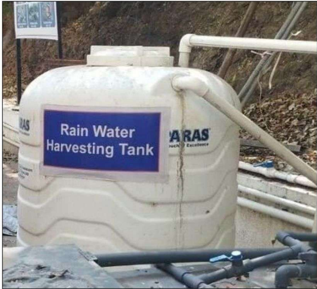
Rooftop Rain water harvesting System
